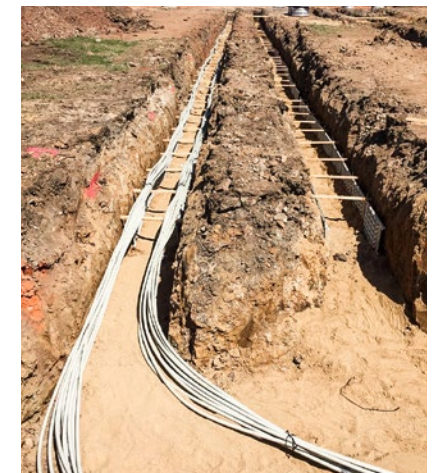
The flow pipes on the one side and the return flow pipes on the other: they are fixed above the collectors.
